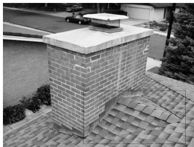
Clay Liner Cover
