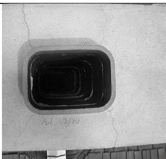
Clay Tile Liner Flue
