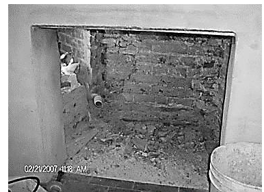
Badly Deteriorated Firebox
