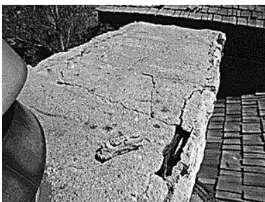
Damaged Chimney Cap
