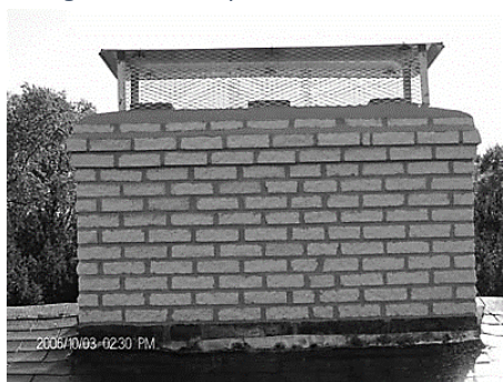
Metal Cap on Clay Liner Chimney Top
