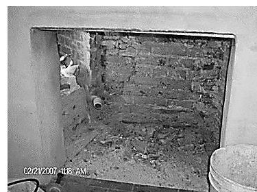
Badly Deteriorated Firebox
