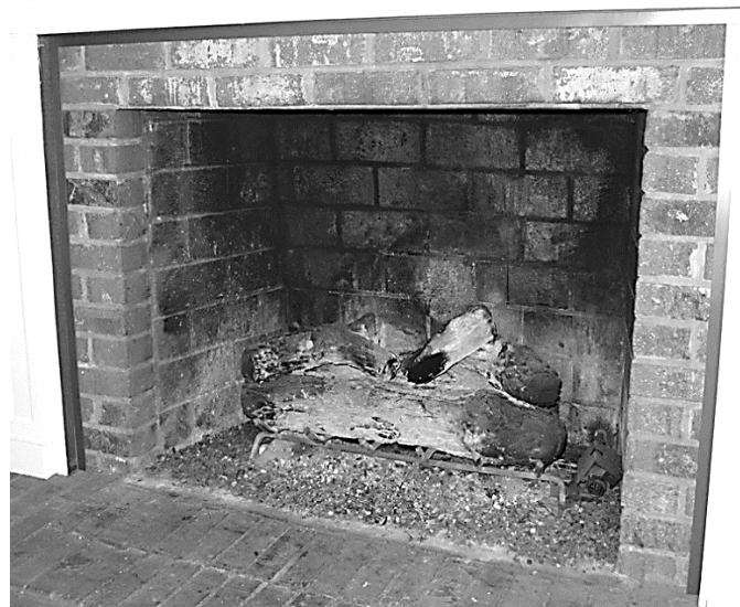
Masonry Woodburning Fireplace
