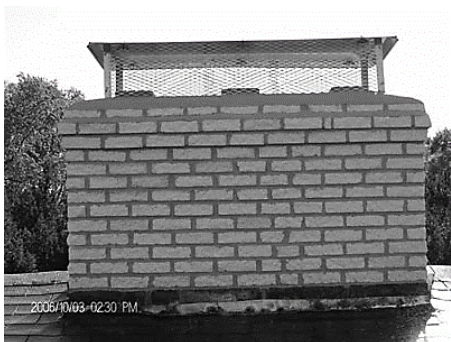
Metal Cap on Clay Liner Chimney Top
