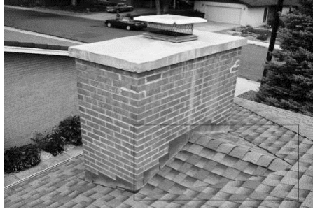
Clay Liner Cover
