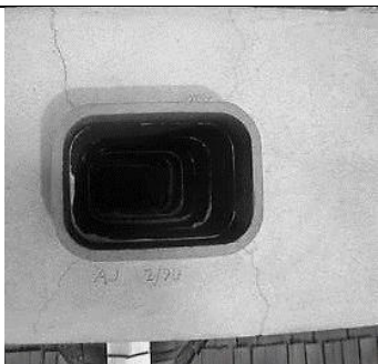
Clay Tile Liner Flue
