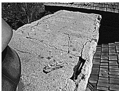
Damaged Chimney Cap
