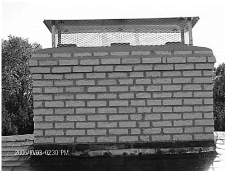
Metal Cap on Clay Liner Chimney Top
