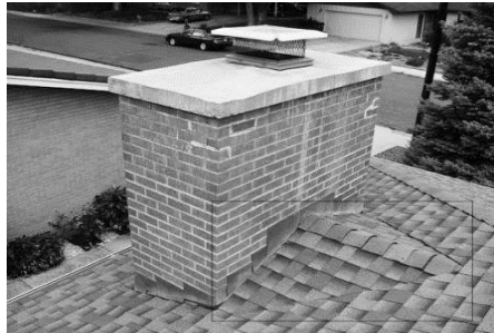
Clay Liner Cover
