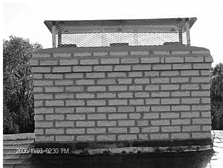
Metal Cap on Clay Liner Chimney Top
