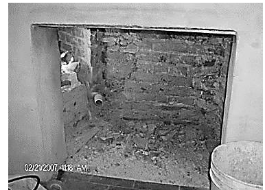
Badly Deteriorated Firebox
