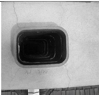
Clay Tile Liner Flue
