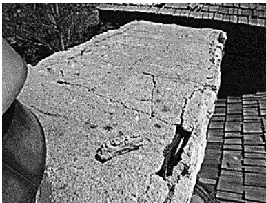
Damaged Chimney Cap
